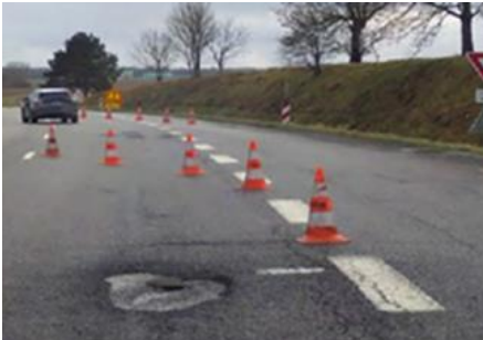
Figure 1: European bituminous road, after winter.
